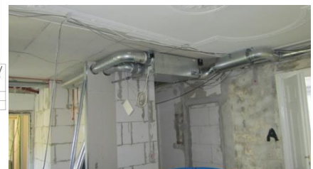
Decentralised HRV in urban renewal in Copenhagen
